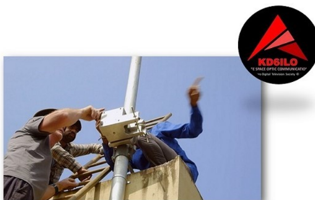
Free Space Optic Communications Transceiver installation San Diego DTV Society members at Carlsbad California Lab.
