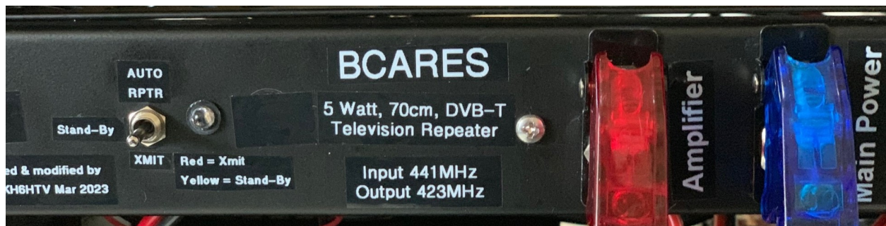
Fig. 7 Main Repeater Controls
